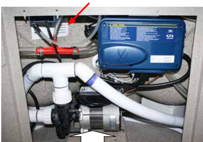
110 Volt Equipment Compartment
